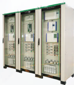
Control & Protection Panel
