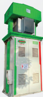
Compact Kiosk Substation
